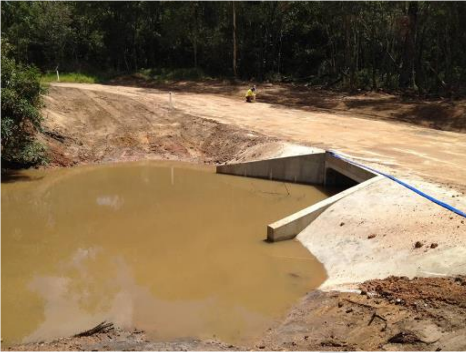
Photo E: Looking at the completed waterway barrier works from an upstream position.
